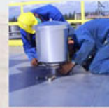
Oil Storage Tank Top Protection
